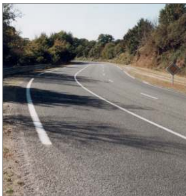
Section with bends: 3 lanes on which overtaking is prohibited in one direction
